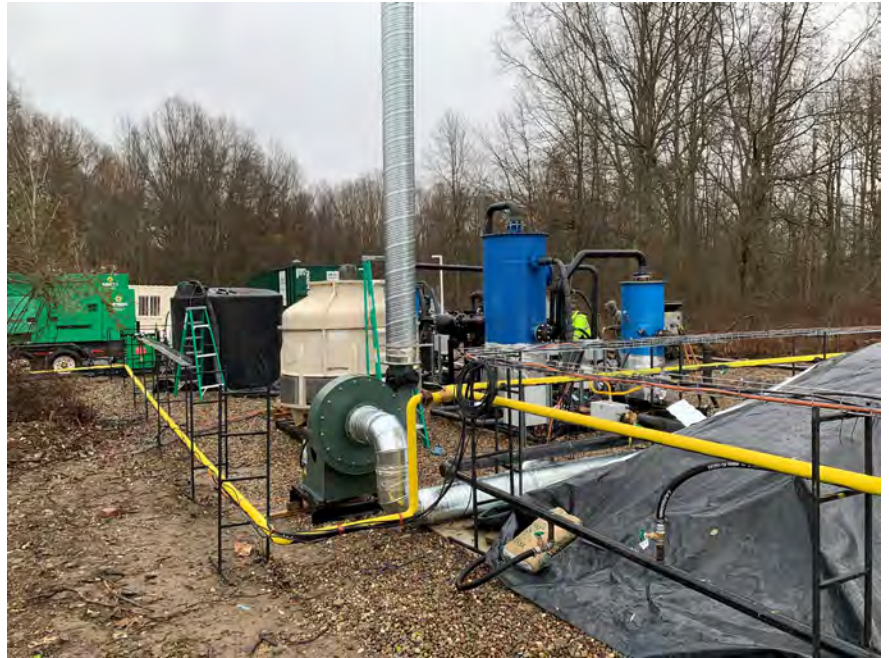
Vapor Treatment System As-Build
