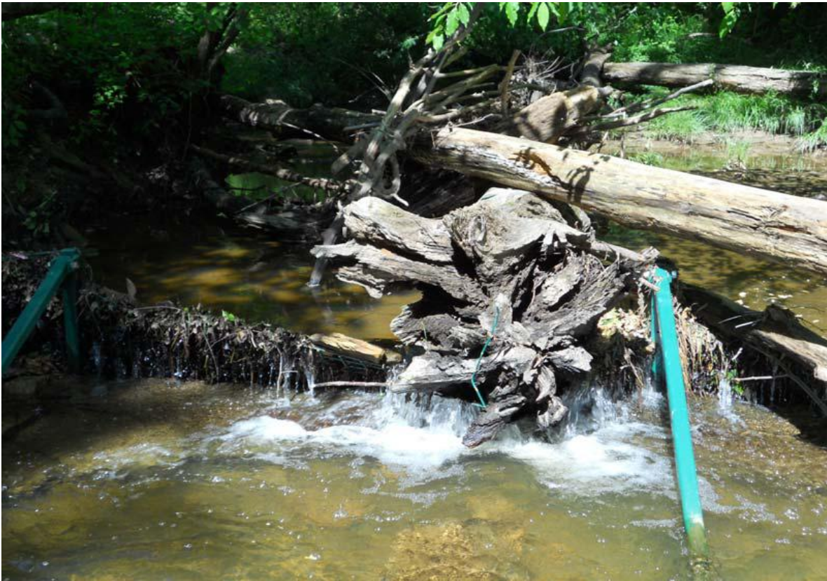
PICTURES SHOWING DAMAGE TO BARRIERS.
