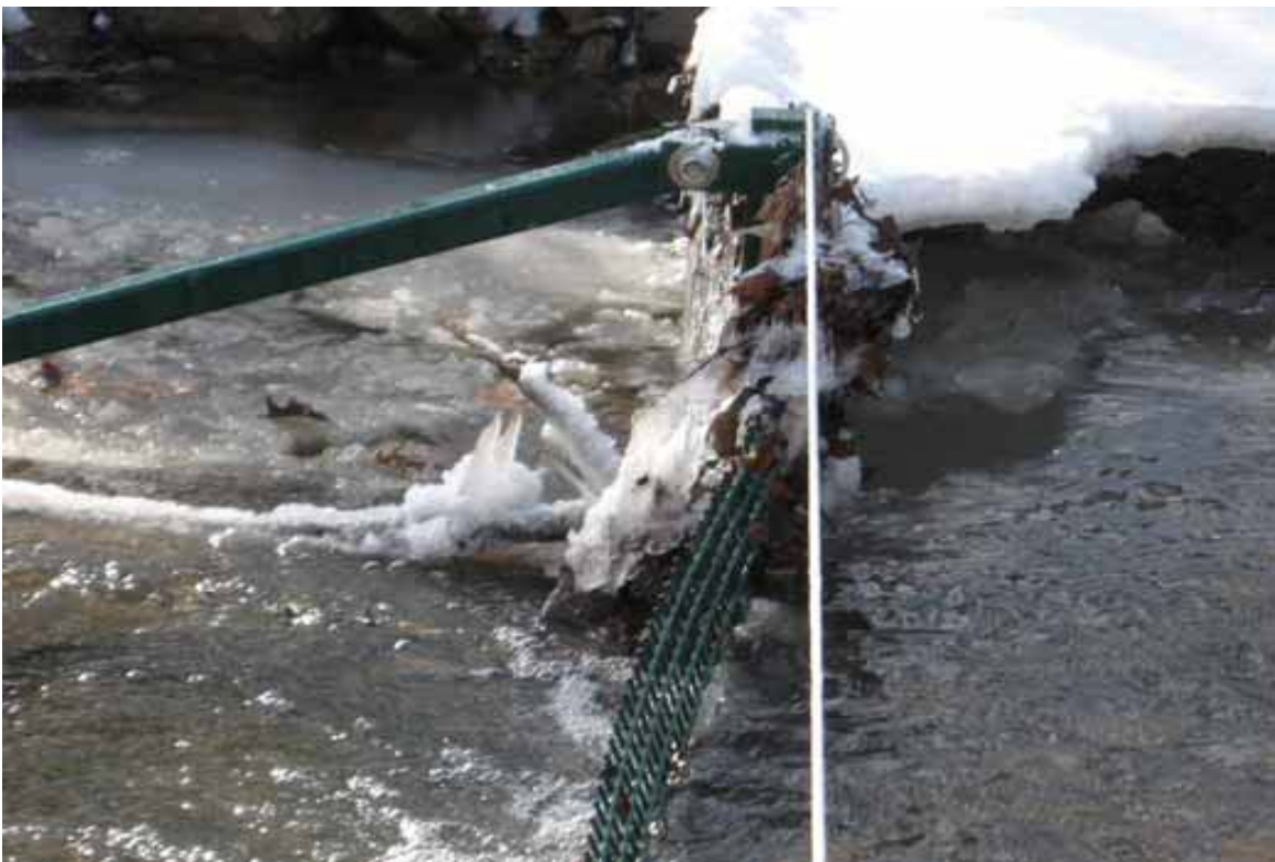
PICTURE SHOWING EXTENT OF BEND IN DOWNSTREAM BARRIER TO DATE.
