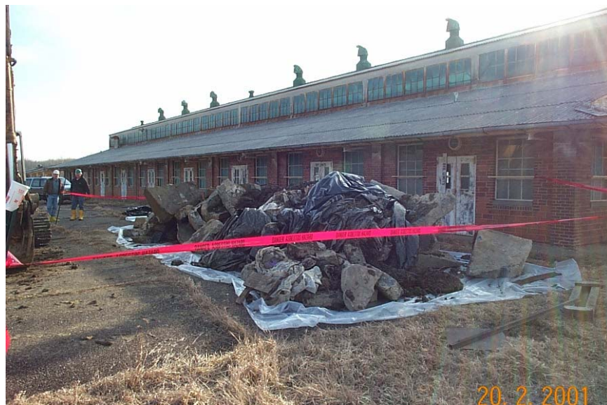
Debris from AP-3, 5, & 6 sumps
