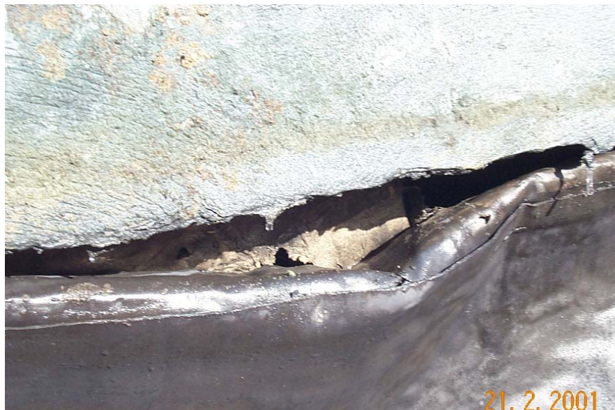
Asbestos Behind Lead Liner
