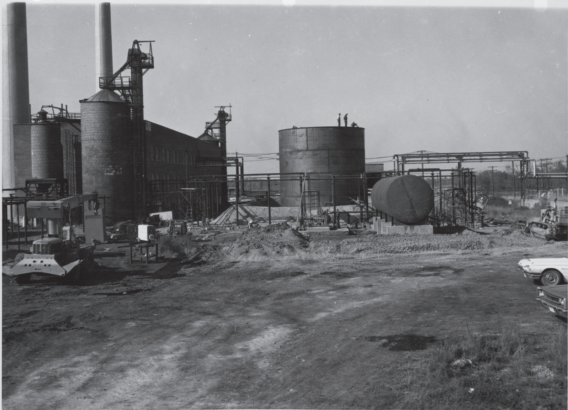
LOUISVILLE DISTRICT, CORPS OF ENGINEERS, U. S. ARMY. Date: 15 October 1968 File No. 40016 Ravenna Arsenal, Ravenna, Ohio. Rehabilitation of shell loading facilities (PEMA), Contract DACA-27-68 C-0045, Blount Brothers Corp., Montgomery, Ala., dated 6 June 1968. Load Line No. 2, Item 20, conversion of boilers power house 3 to oil fired showing oil storage tanks and piping.
