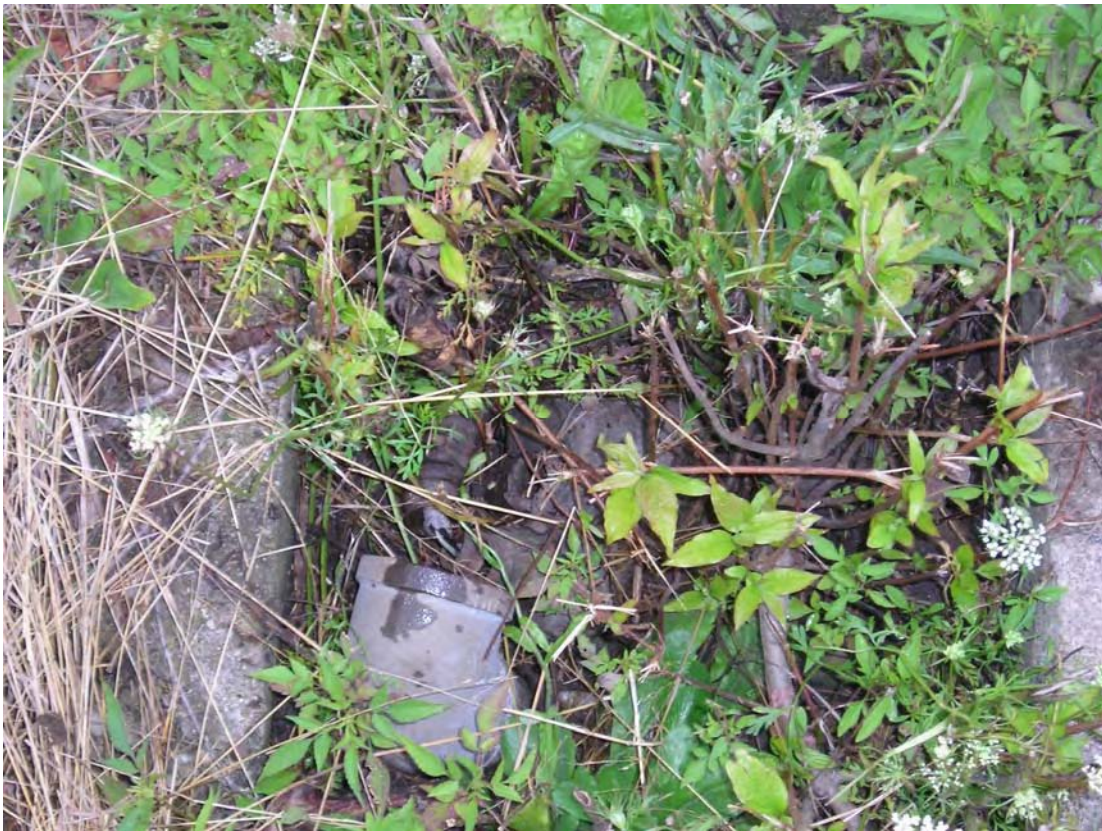
Photograph 3: Pipe and electrical wire at Site 1.
