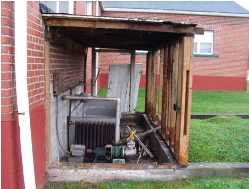
Laundry Flame Proofing Building prior to demolition. Portion of sump visible on right. Sump was filled with clean soils during past closure activities by the facility. Sump soils to be re-used for backfill during restoration operations.
