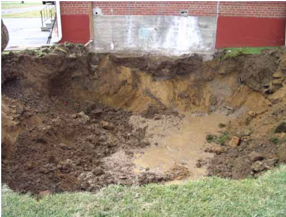
Picture showing resultant excavation following removal of floor slab and adjacent sump.
