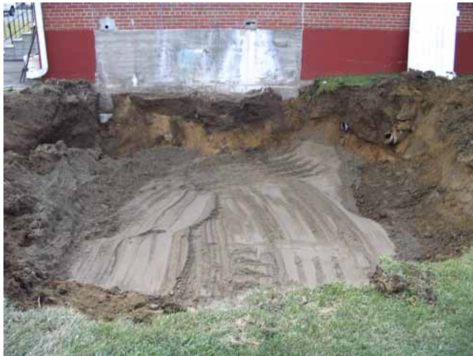
Picture showing the layer of clean sand installed (per scope of work) for use as a marker during future investigation and sampling operations under separate contract.
