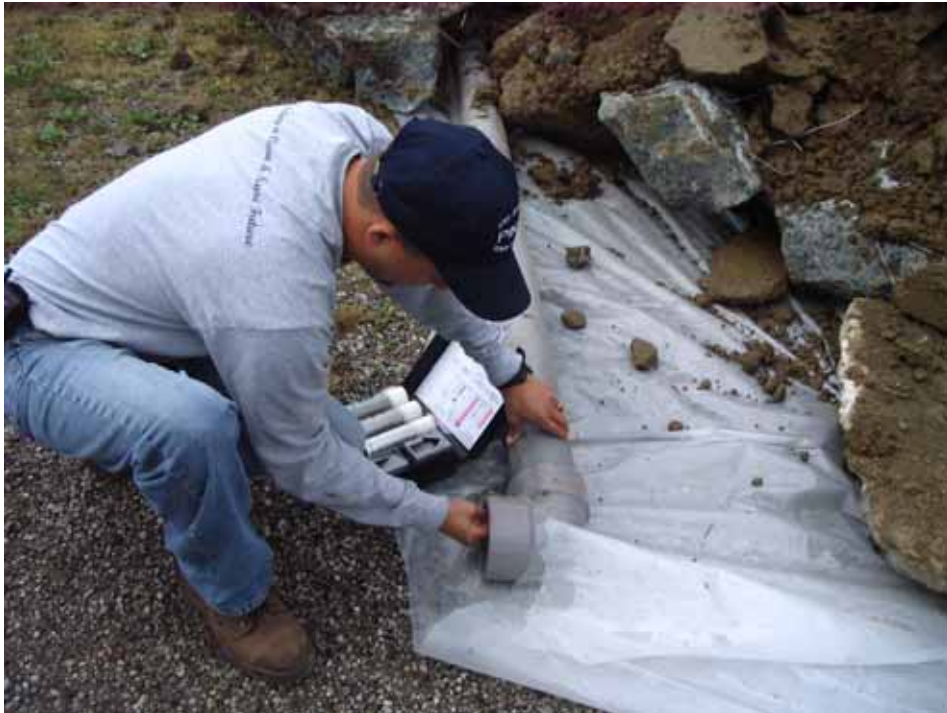
Expray testing building piping to verify no explosives present. Expray results are negative.
