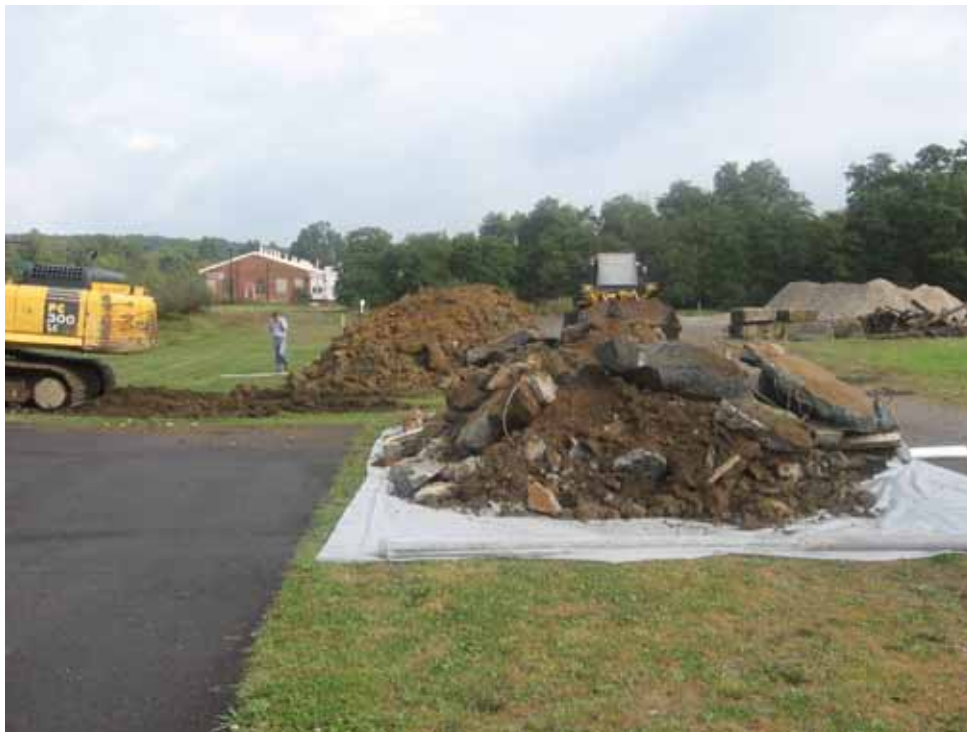
Close-up of staging area for demolition debris. Clean soils (background) from inside sump staged for re-use as backfill as per scope of work.
