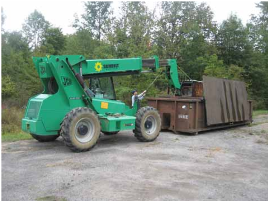
Transferring inspected and certified scrap metal and MDAS into lockable rolloff for subsequent recycling at off site smelter facility.
