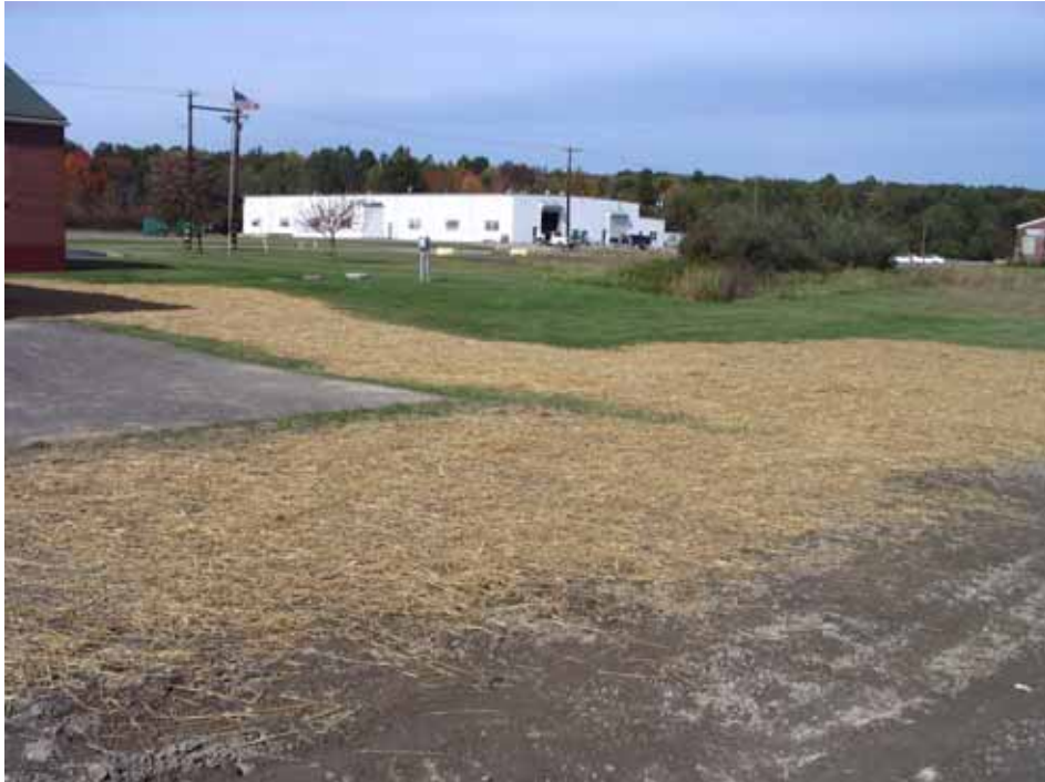
Picture showing Laundry Flame Proofing Building area following removal of demolition debris and final grading, seeding and mulching.
