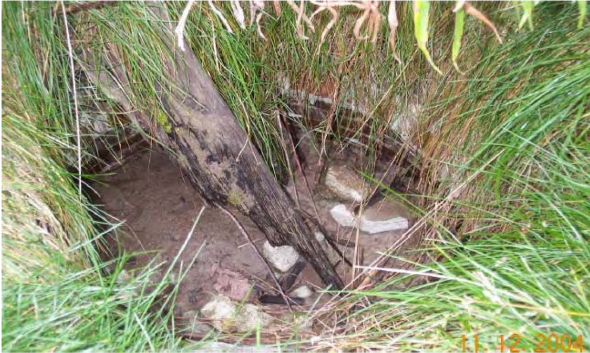
035 - Sewer at Atlas Scrap Yard with no lid and full of surface debris, no sample was collected from this sewer location.
