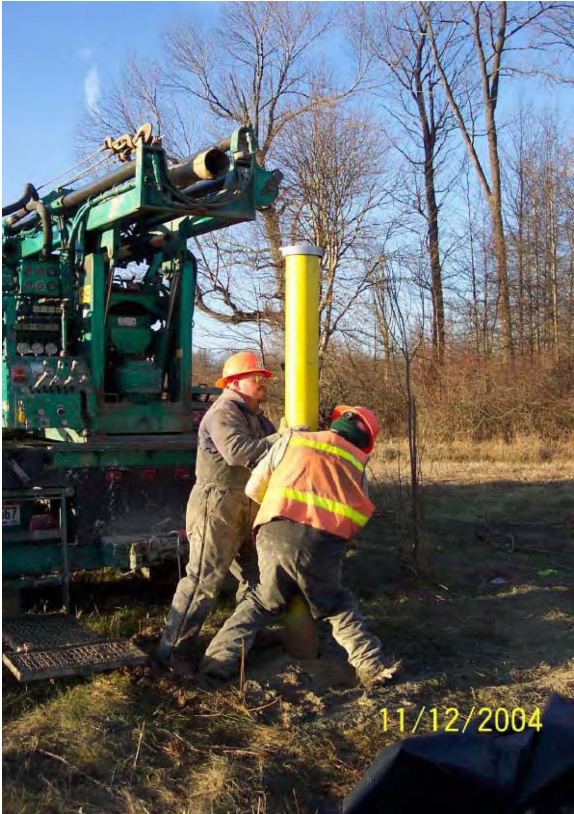
052 - Installing pro-casing over the inner casing of a monitoring well at Atlas Scrap Yard.
