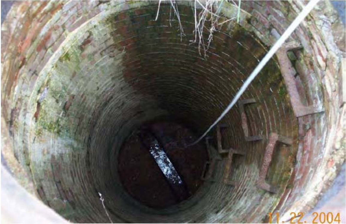
025 - Silicone tubing lowered into water channel from sewer at LL 7-Sewer was approximately 18 ft. deep and the water level in the channel was approximately 1 in. deep.
