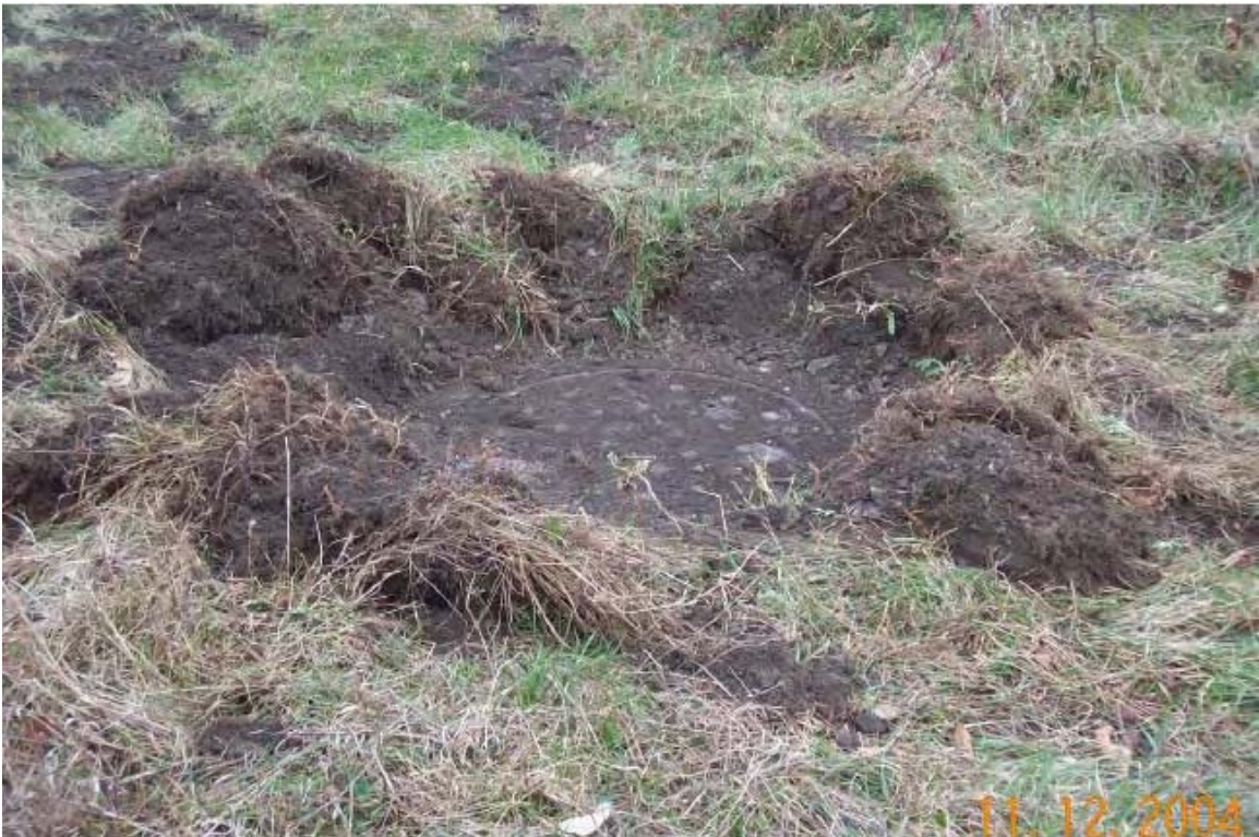
032 - A buried sewer at Atlas Scrap Yard located using magnetometer and referencing site maps.
