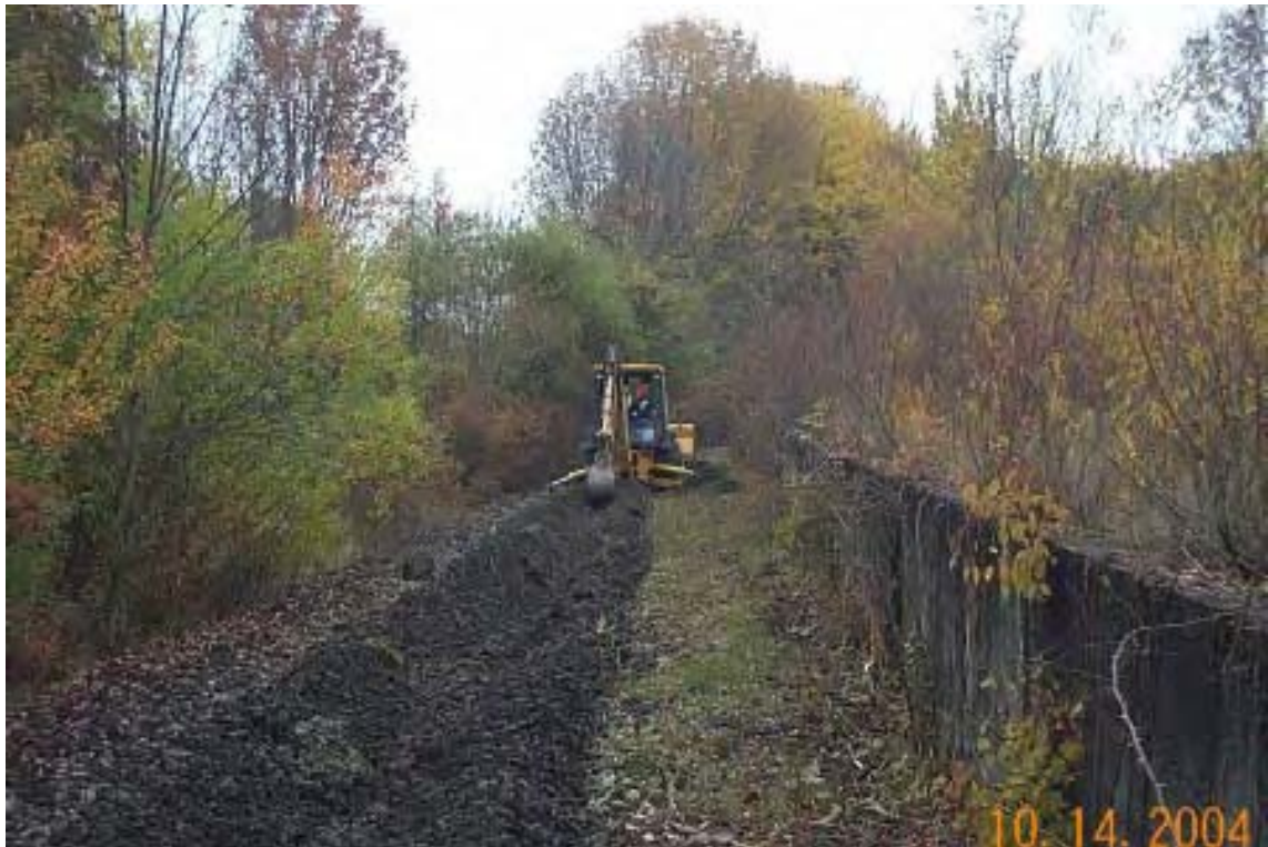
008 - Trenching the center of the railroad bed to expose the underlying soil for MI sampling at F15/F-16.
