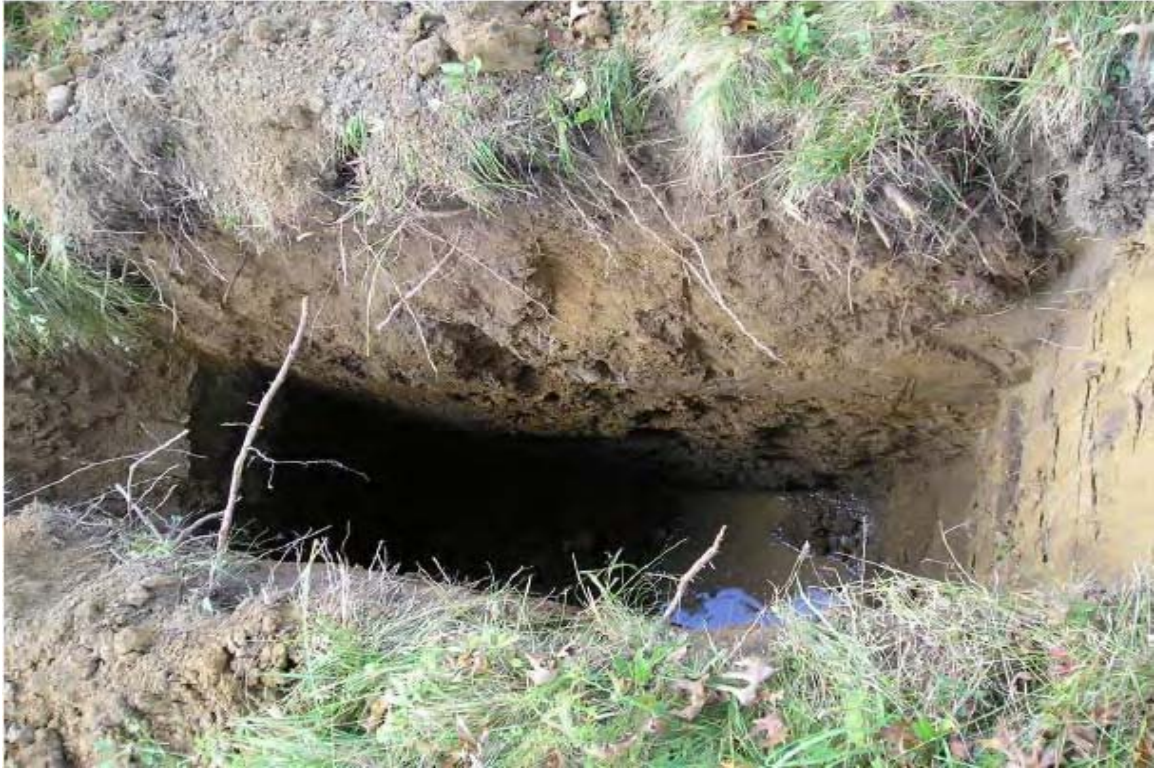
007 - Trench excavation at NACA Test Area. (water present at bottom of trench)
