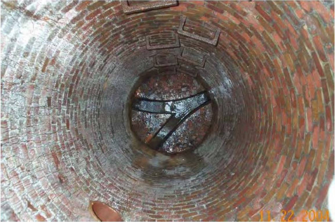
029 - View of a sewer at LL 7 ( \approx 21 ft. bgs) –Water level in channel \approx 2 in deep.
