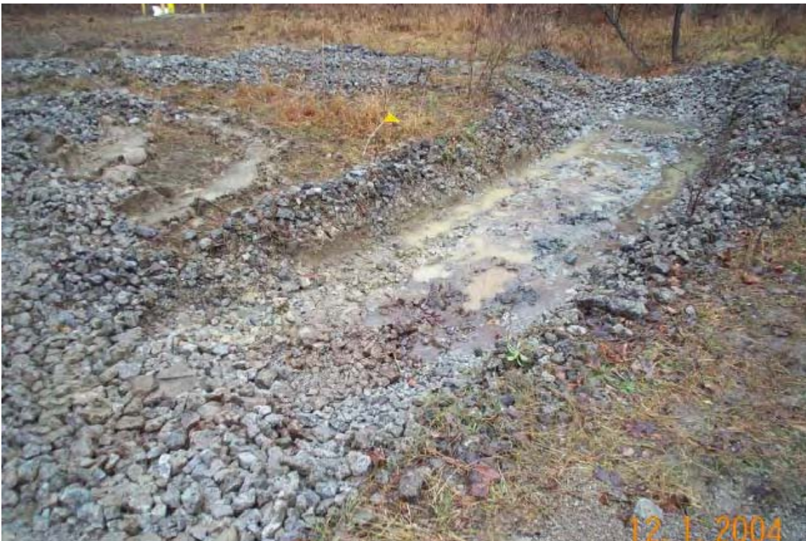
020 - Scoped as a shallow soil MI dry ditch at Building 1200. Ballast was removed prior to sample collection.
