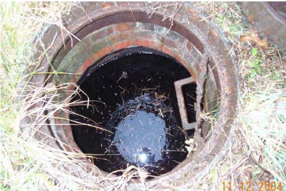
030 - Sewer at Atlas nearly full of water.
