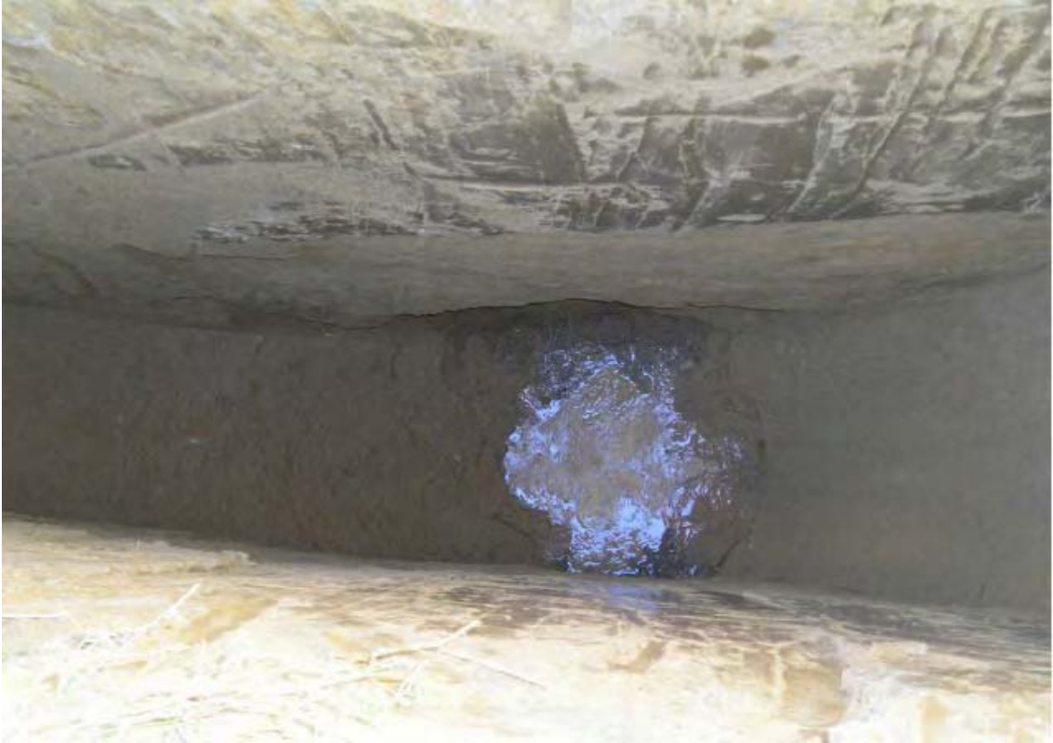
006 - Trench excavation at Atlas Scrap Yard. (water present at bottom of trench)
