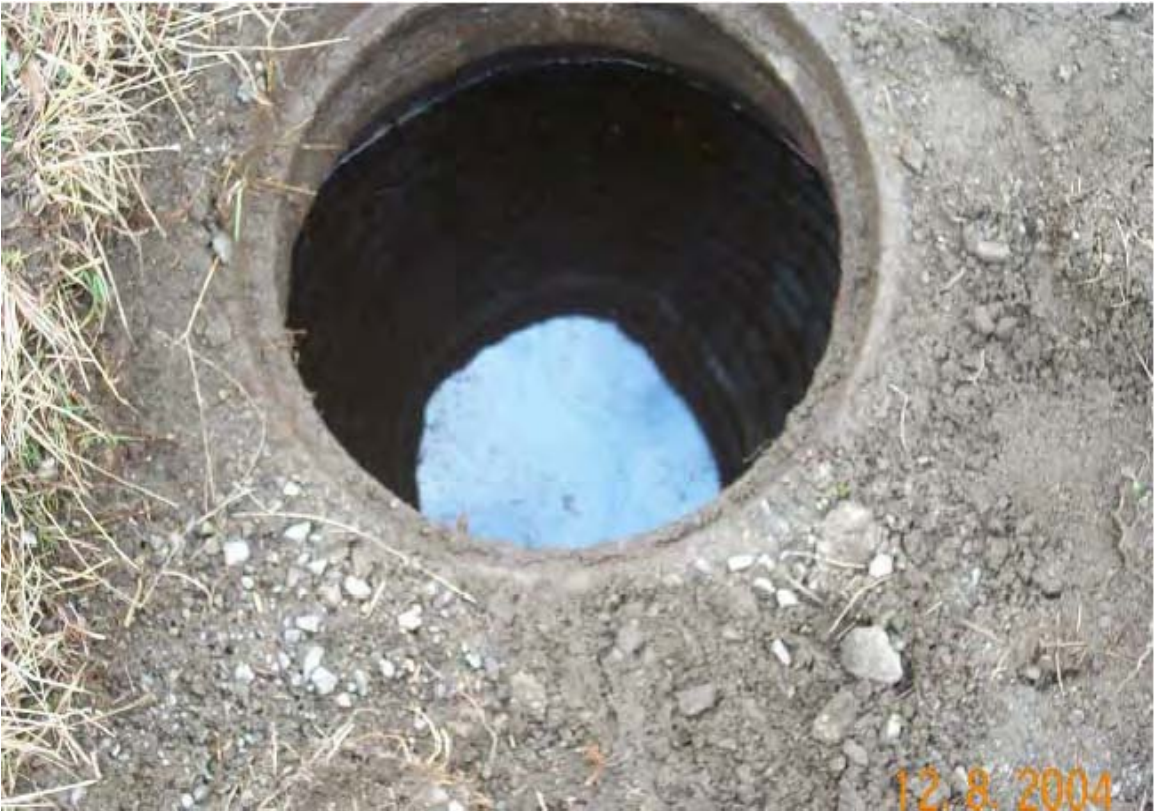
028 - Sheen on sewer water in sewer #10 at Atlas Scrap Yard.
